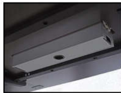
Comms Box (underneath)
